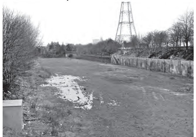
The cleared High Level Station site. A lone figure can be seen heading for the railway tunnel. Photo reproduced by permission of Tony Harden from his collection
